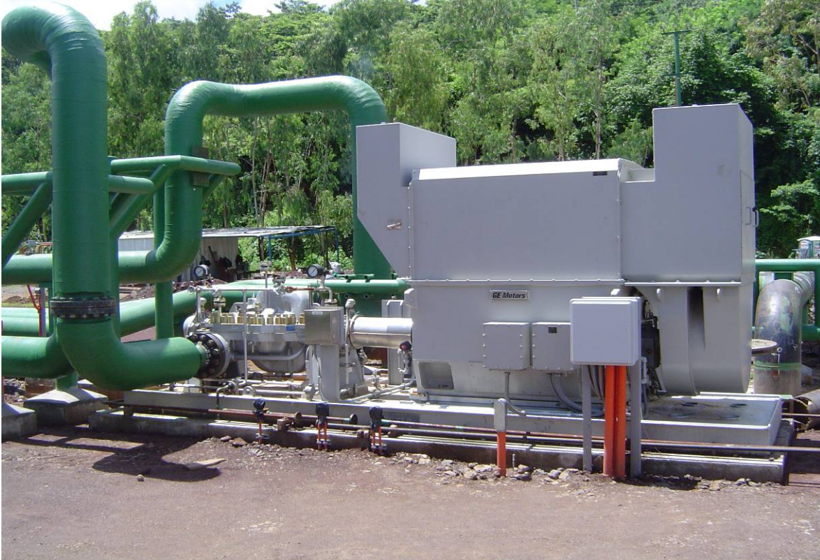
Figure 12 - View of injection pumping system at Berlin Geothermal field, in El Salvador.
