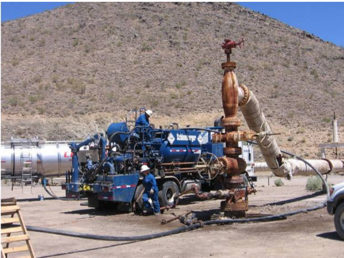
Figure 10 - Installation of a pumping unit for injection of chemical compounds at Coso geothermal field (photo P. Rose, EGI, Univ. of Utah).
