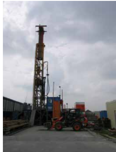
Geothermal well Bleiswijk, NL.
