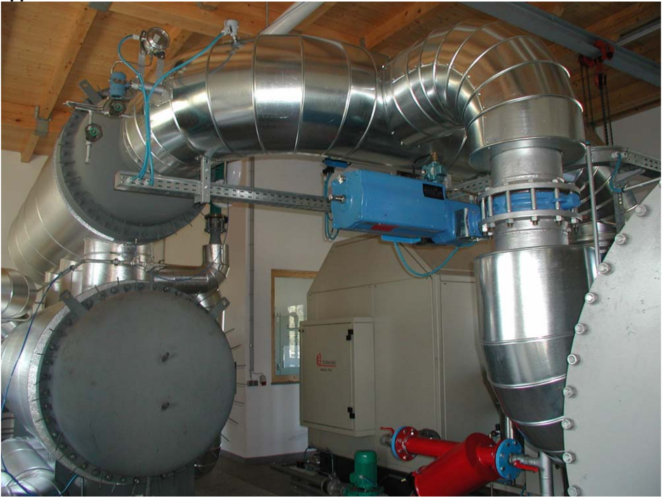
Figure 1 : View to the evaporator, demister, vapour pipes and generator
