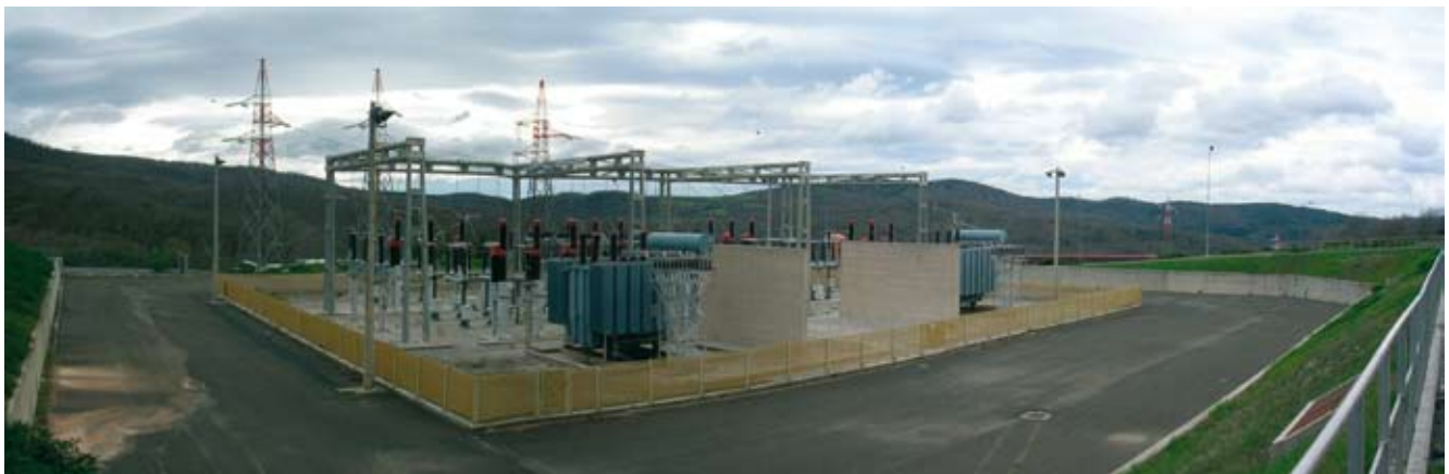
Fig. 3: Part of geothermal power plant of Larderello – Italy (120 MWe capacity)
