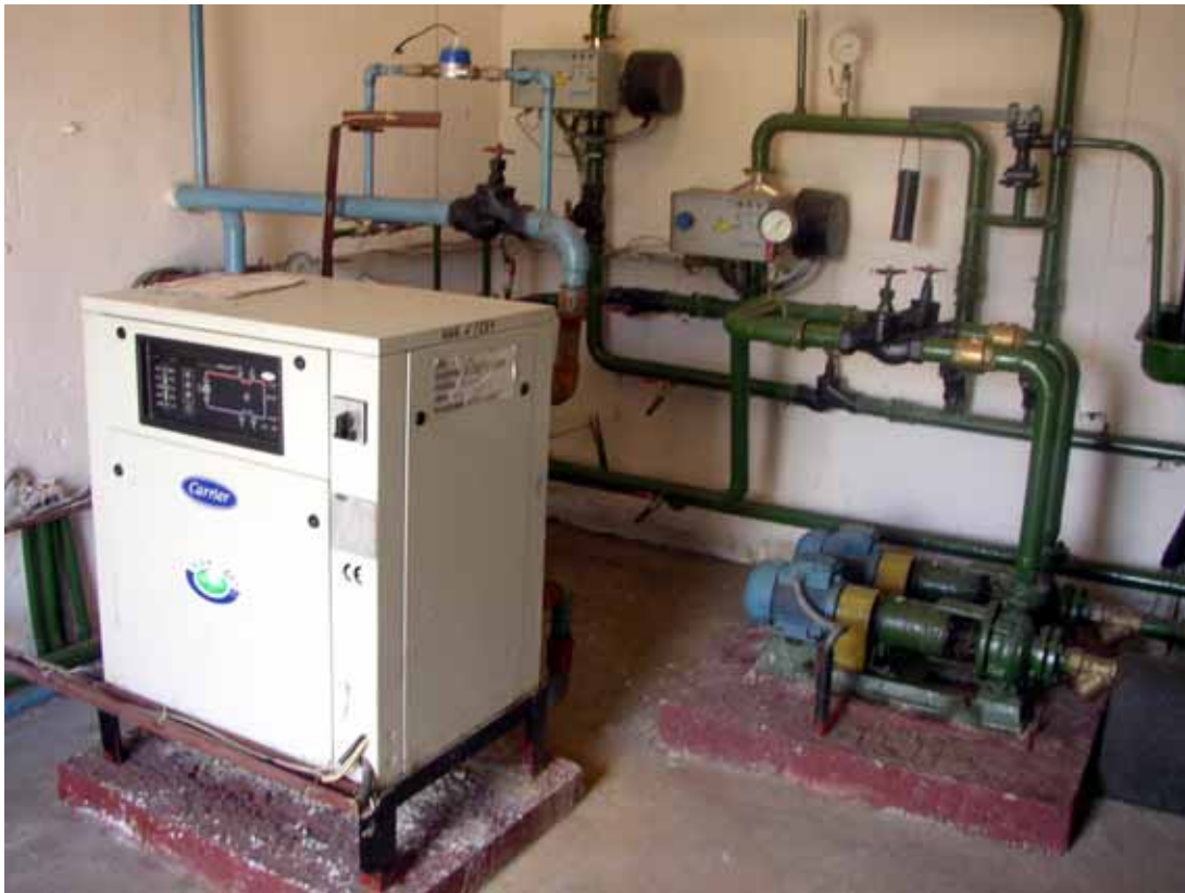
Fig. 2 – A Heat pump installation at one of waterworks located in the Minsk District, Belarus (photo done by I. Zhidovich).
