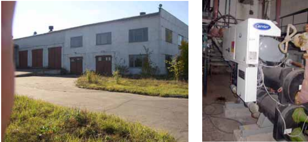
Fig.1 – A heat pump in the process of its mounting (to the right) based on the utilization of a primary heat source, taken from the river water and the building (to the left) heated by this heat pump system (photo done by I. Zhidovich).
